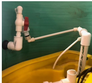
Discharge assembly in septic tank riser
